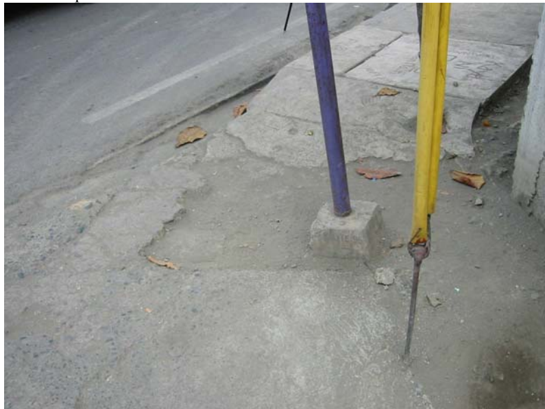
BLLM1 should be positioned where the concrete is broken
